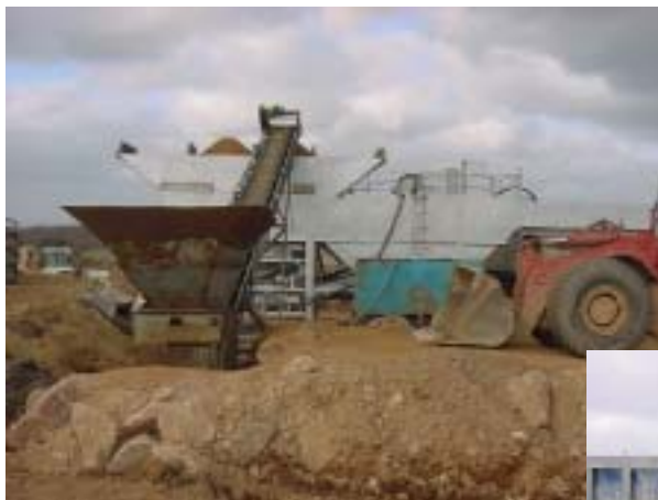
The cement batching plant at SLS
